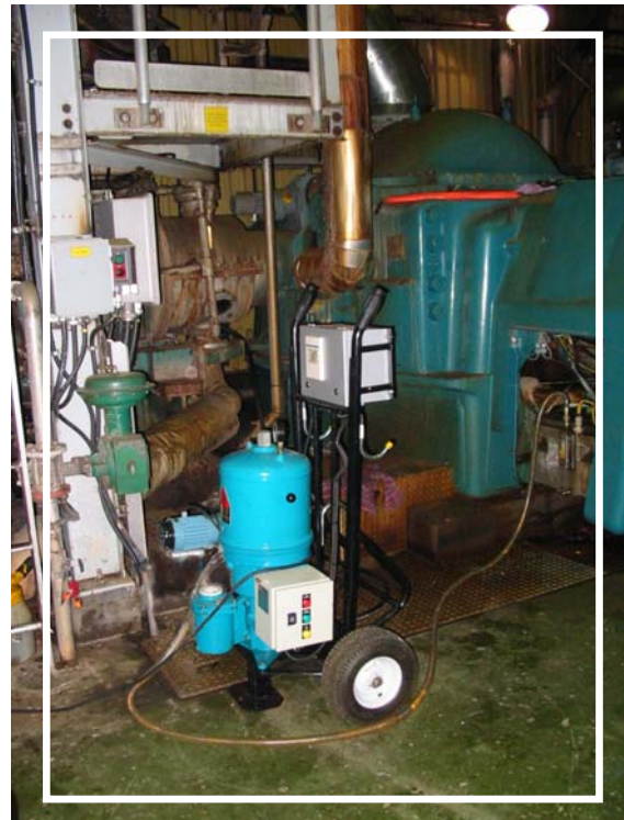
PTU2 27/27 PV-EW on Sunds Refiner
