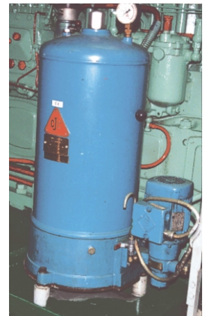
HDU2 27/54 P for lube oil treatment
