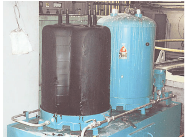
Changing the first set of elements in the HDU 2 x 427/81 MZ-EPQTVY on the 40,000 litre system
