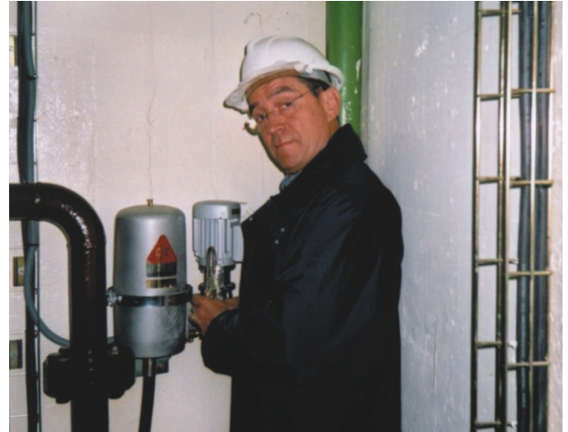
Mr. Jesus Javier Moises in the hydro-electric generation station, next to the CJC™ LG 15/25 L FineFilter.
